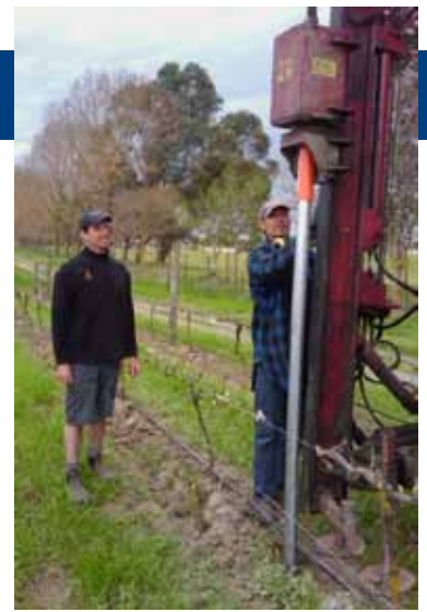
Johnathan Hamlet, Villa Maria's Joseph Soler vineyard manager, looks on as Trevor Manual of VinMan installs the Eco Trellis posts.
